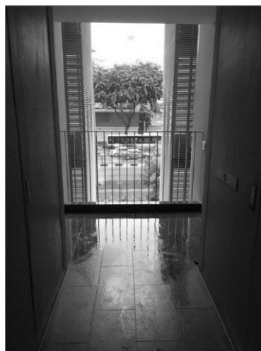
Figure 7: Railing as safety barriers resulting in extensive wind-driven rain into corridor
