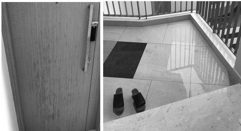
Figure 1: Examples of deterioration to door material and ponding along the corridor
